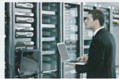
Security Control Systems
