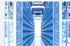
Data System Rooms
